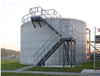
Figure 1 – Full-scale BAC filter at Puurwater Fabriek , Emmen, The Netherlands 4 .
