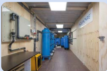
BioPhree installation. Picture: Aquacare
