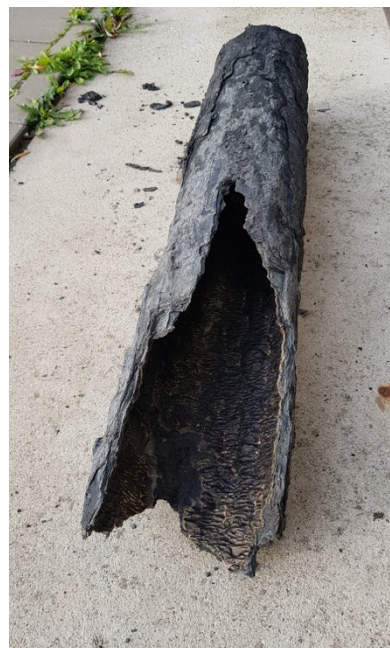
Vivianite scaling in a sewage pipe
